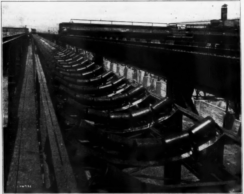
Detail View of the Ball Bearing Troughing Idler Pulleys
